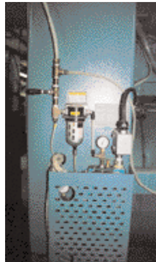
Washing machine air feed supply
