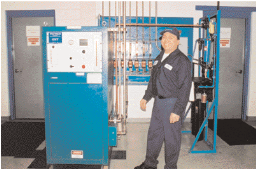
Plant Supervisor Nino Velez oversees the ozone injection system (at left) at Clean Rentals Inc., a company specializing in uniforms and shop towels. Velez says the ozone system has improved wash quality, while saving on water and chemical use.
