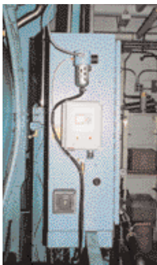
A satellite reader that allows employees to track the use of ozone in an individual washing machine.
