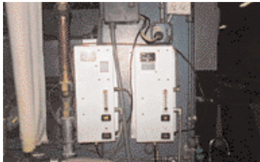
A close-up view of the ozone units on the Acme washer
