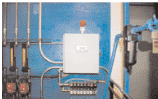
Wastewater and wastewater are treated by this ozone system.
