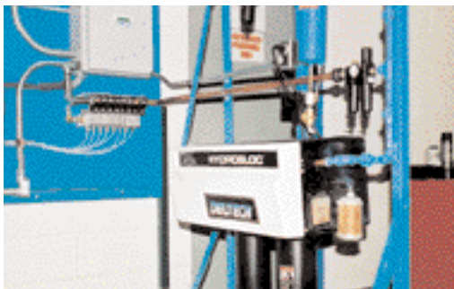
A section of the ozone injection system at Clean Rentals
